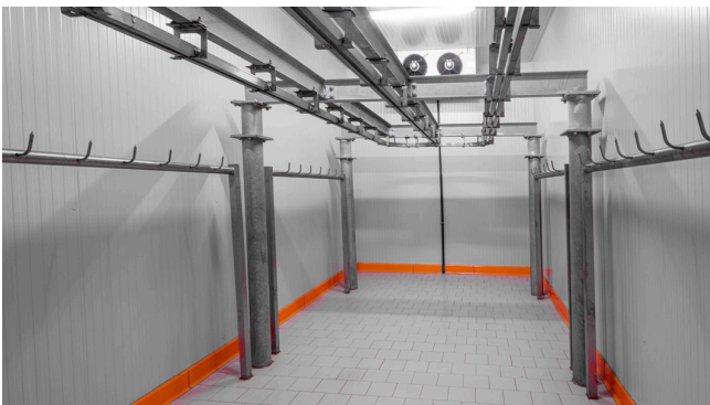
Cold Room and Storage
