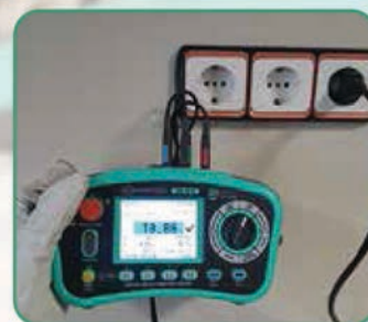
Loop test from a wall socket
