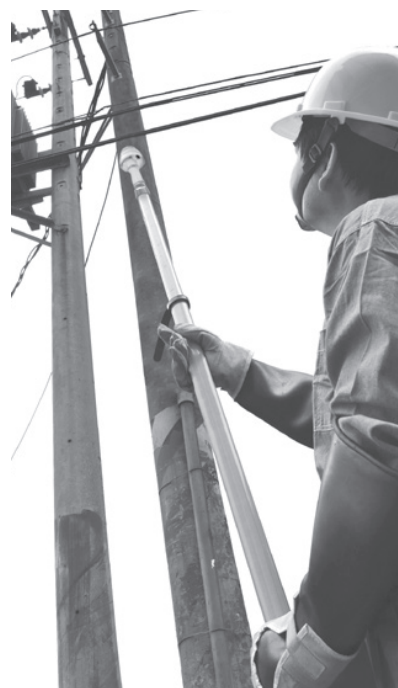
Fig. 3: Voltage detection for overhead lines
