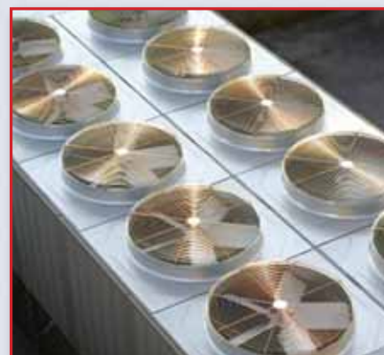
Rooftop HVAC System
