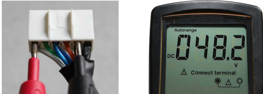
Test Connection between Clamp 1 & Clamp 5 of 12V Cells
