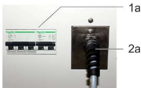
Safety cutouts and mains cable at W80t
