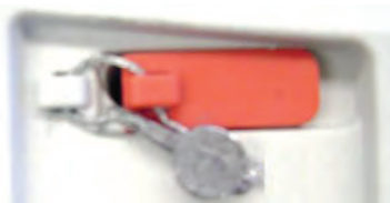
Locked with Wire Seal
