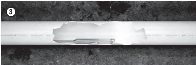
3 RE-INSPECT THE LINE TO ENSURE IT IS FREE OF DEBRIS AND CONFIRM LOCATION AND SIZE OF REPAIR
