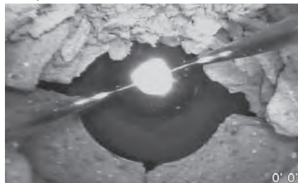
Figure 13 – Typical Crossbore Into Sewer Line
