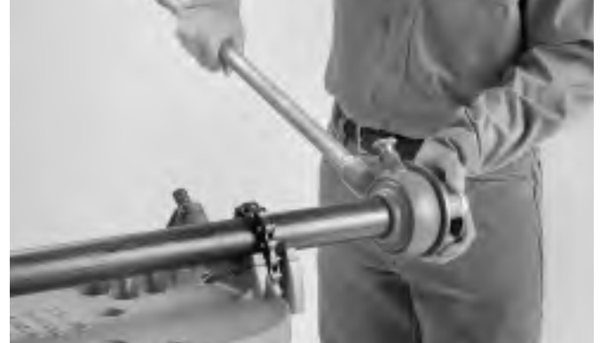
Figure 3 – Sliding Threader On Pipe
