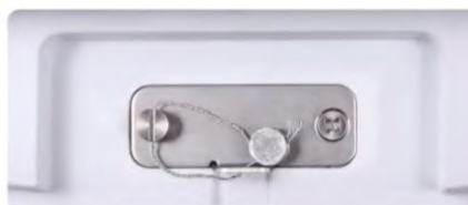
Locked with Wire Seal
