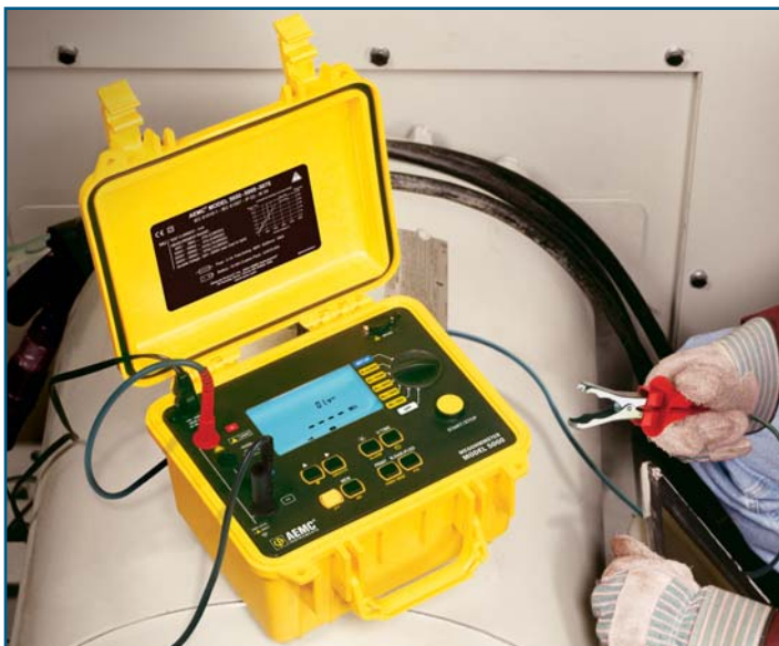
Model 5060 performing insulation test on a generator.
