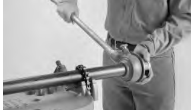
Figure 3 – Sliding Threader On Pipe
